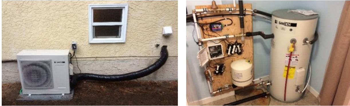
Figure 41: Kelowna Site 1 Installed Photos
