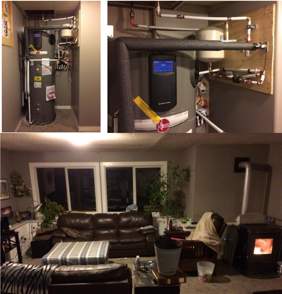
Figure 50: Kelowna Site 3 Installed Photos – Unducted System in Condition Space
