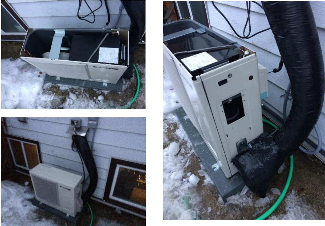
Figure 35: Rossland Site 3 GS3 (New) Unit Installation Photos
