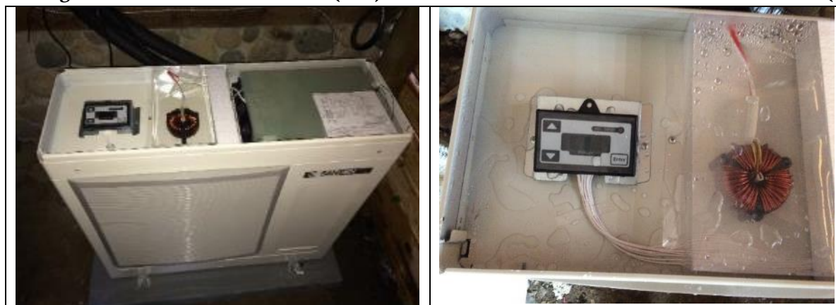
Figure 28: Normal controller (left) and Condensation in Unit from Infiltration (right)
