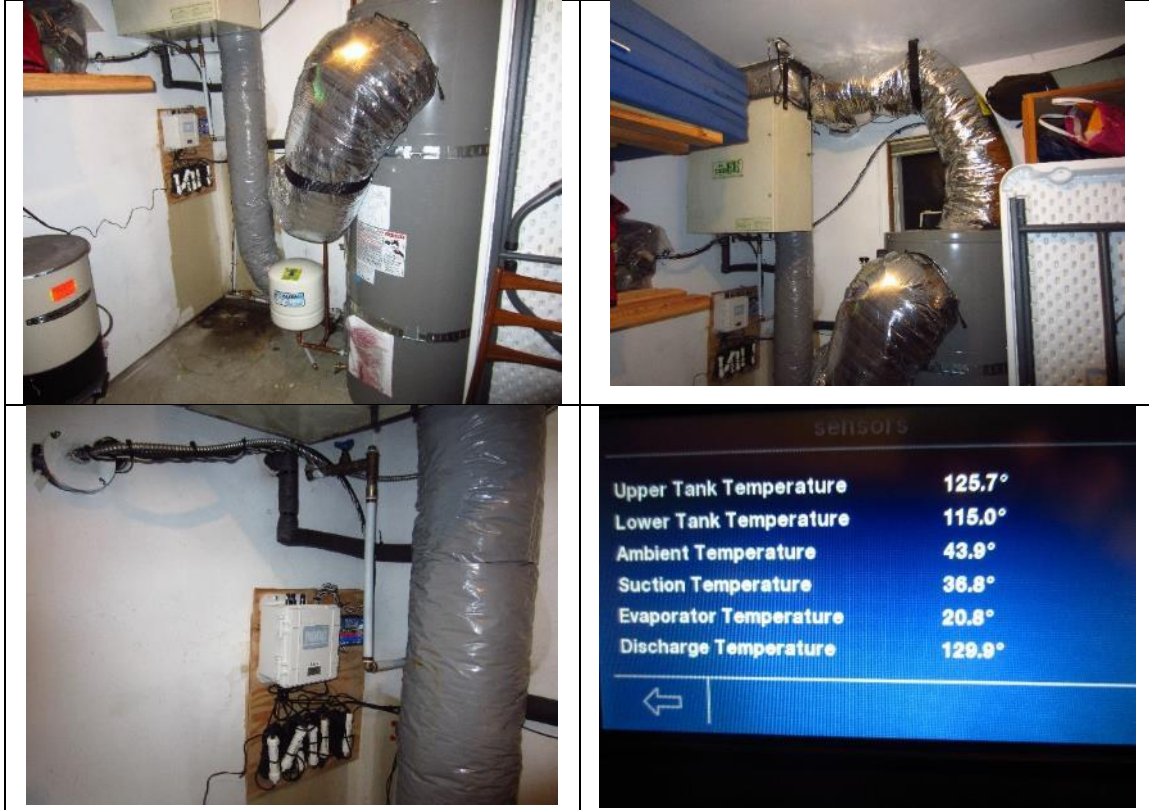
Figure 56: Vancouver Island Site 1 Installed Photos
