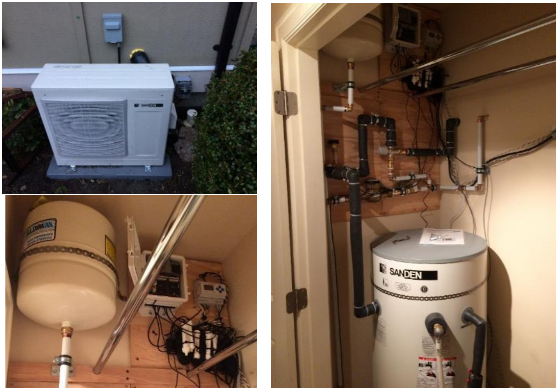
Figure 45: Vancouver Island Site 2 Installed Photos
