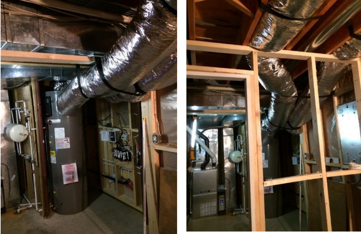
Figure 54: Kelowna Site 4 Installed Photos
