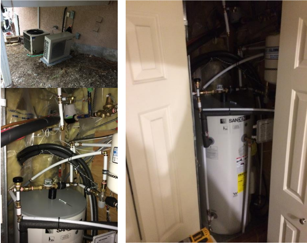
Figure 43: Kelowna Site 2 Installed Photos
